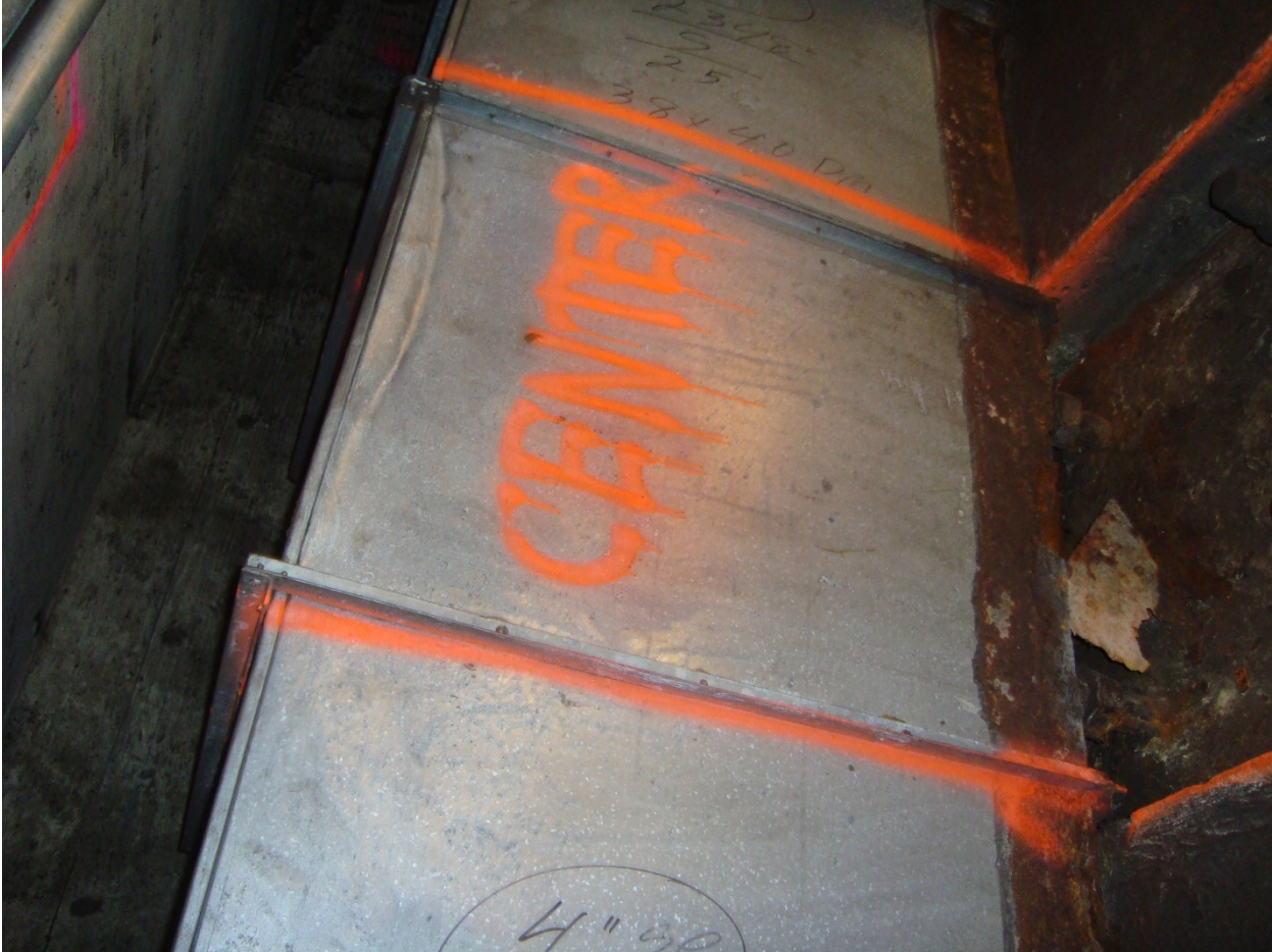
22-Bethesda Plenum, 5'X2' Mezz. column, looking down, 8-2-2015
