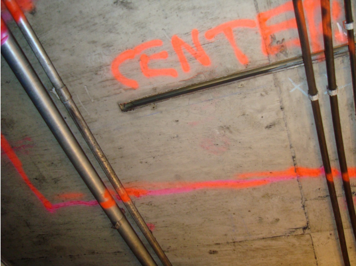
20-Bethesda Plenum, 5'X2' Mezz. column, looking up, 8-2-2015
