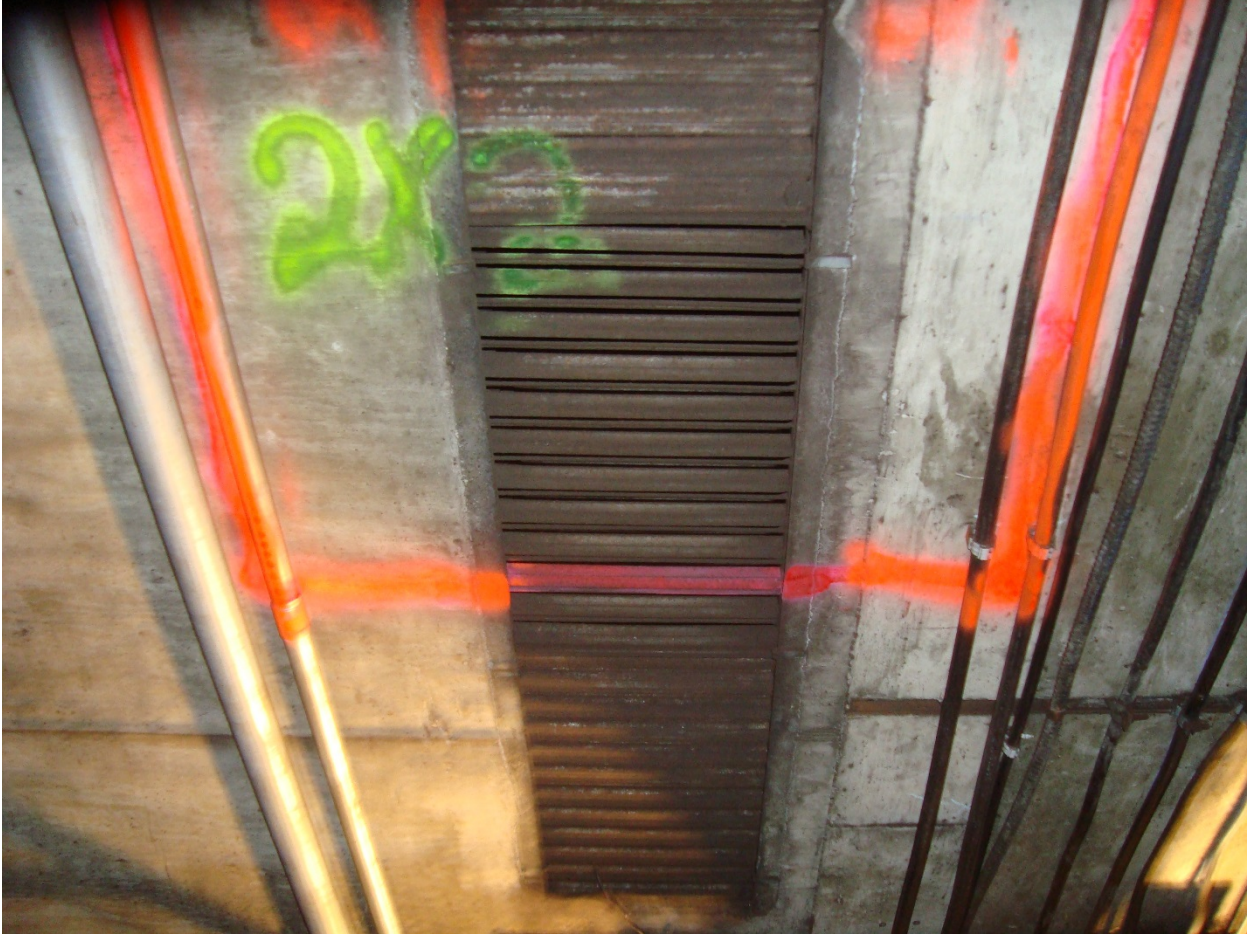
14-Bethesda Plenum, 2'X2' Mezz. Column, looking up, 8-2-2015
