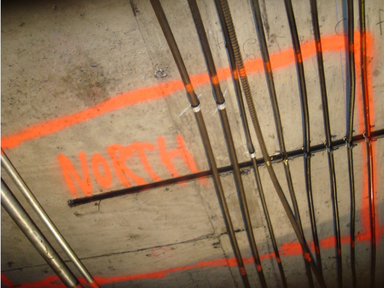
32-Bethesda Plenum 5'X2' Mezz. column looking up, 8-2-2015
