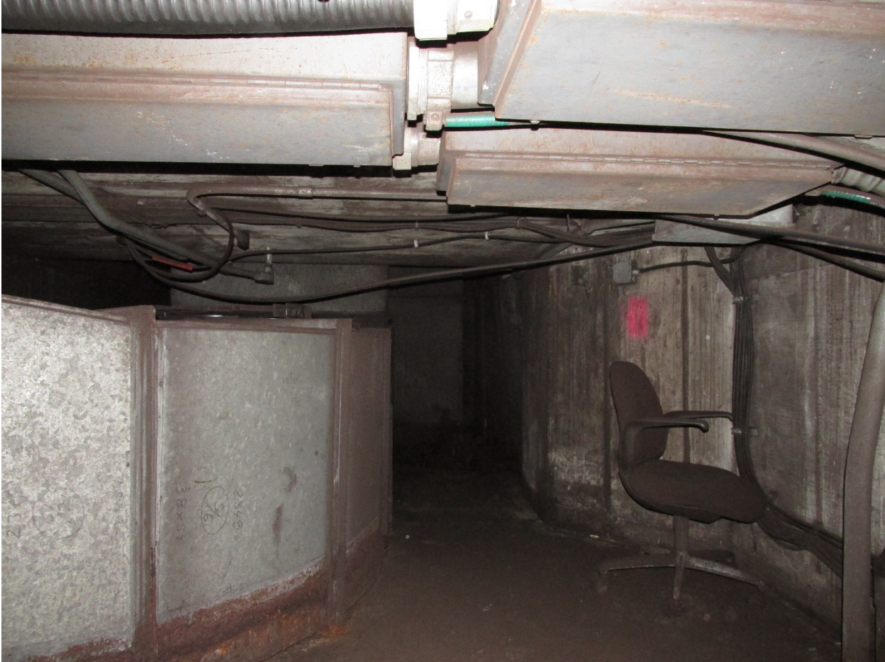
A09 Platform South Side Plenum Inbound Side looking south
