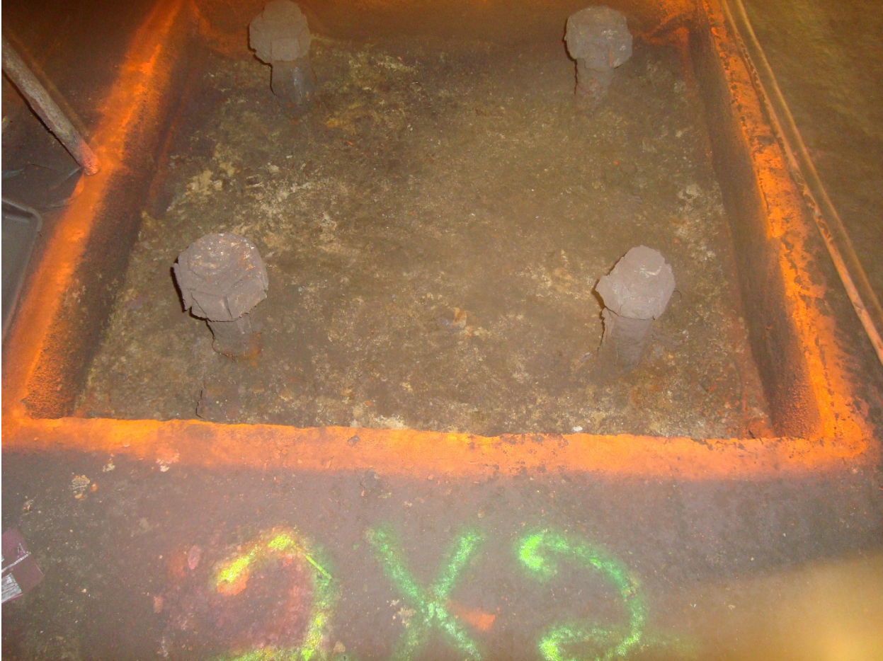
15-Bethesda Plenum, 2'X2' Mezz. column, looking down, 8-2-2015
