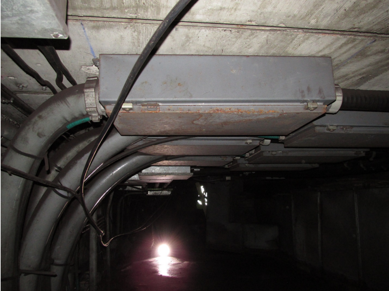
A09 Platform South Side Plenum Inbound Side looking north
