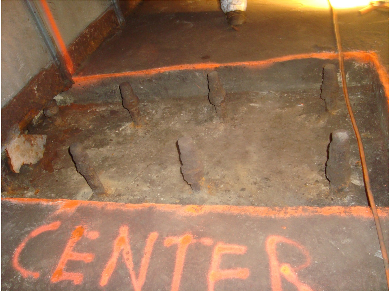
23-Bethesda Plenum, 5'X2' Mezz. column, looking down, 8-2-2015
