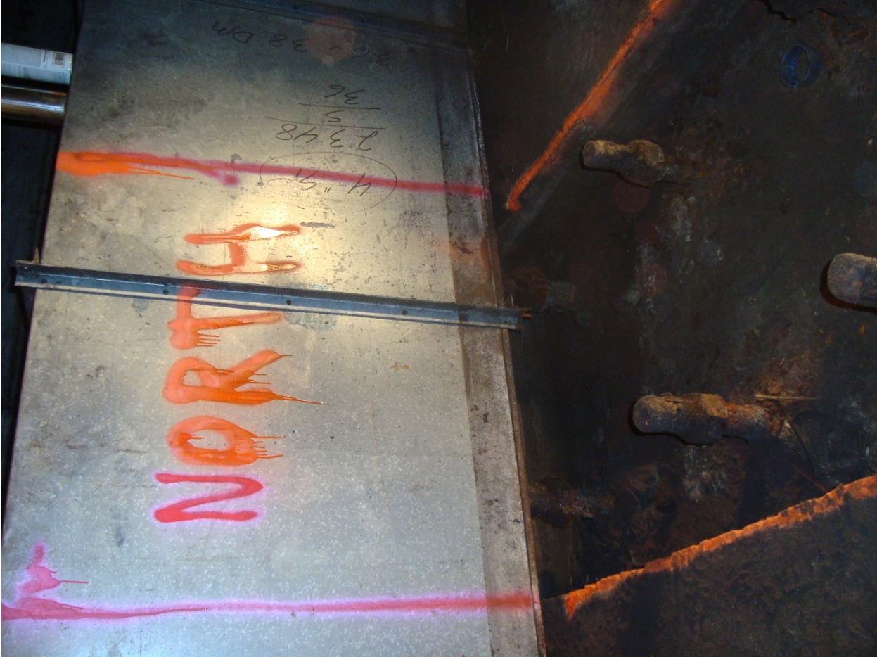
31-Bethesda Plenum 5'X2' Mezz. column, looking down, 8-2-2015
